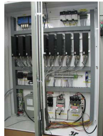
Multiple V84i controllers in PLC enclosure
